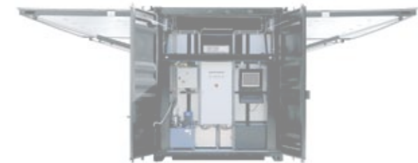
A view of the technical room in the Crowd Gate. All the control components easily accessible and securely locked behind steel doors.
