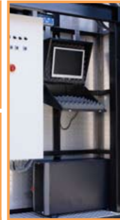
The Crowd Gate control room houses a server which can manage up to 60 turnstiles and send real-time data to other computers in the network or via the internet.
